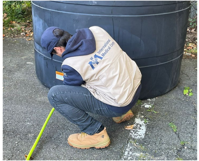
A staff member connects a water source to a 1,000 gallon water tank after delivering it to an FQHC facility in Asheville, North Carolina.
