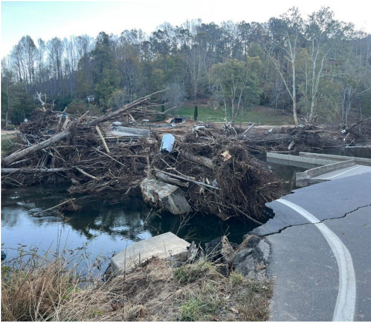
Road damage from flooding in Buncombe County, North Carolina, following Hurricane Helene.
