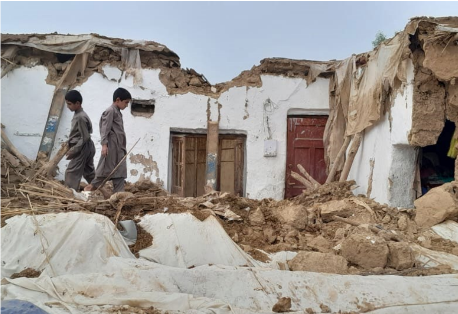
A house damaged by the recent flooding in Khyber Pakhtunkhwa province, Pakistan.
