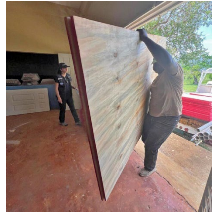
Local workers retrofit the Barbary Community Center, in St. Elizabeth Parish, Jamaica, as a temporary health facility, due to severe damage caused by Hurricane Beryl.
