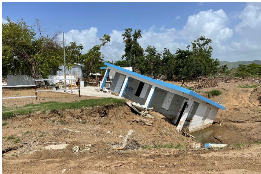
A house in Salinas, Puerto Rico, that was destroyed by flooding and mudslides during Hurricane Fiona.
