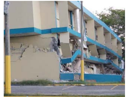
Damage to school in Guanica, Puerto Rico.
